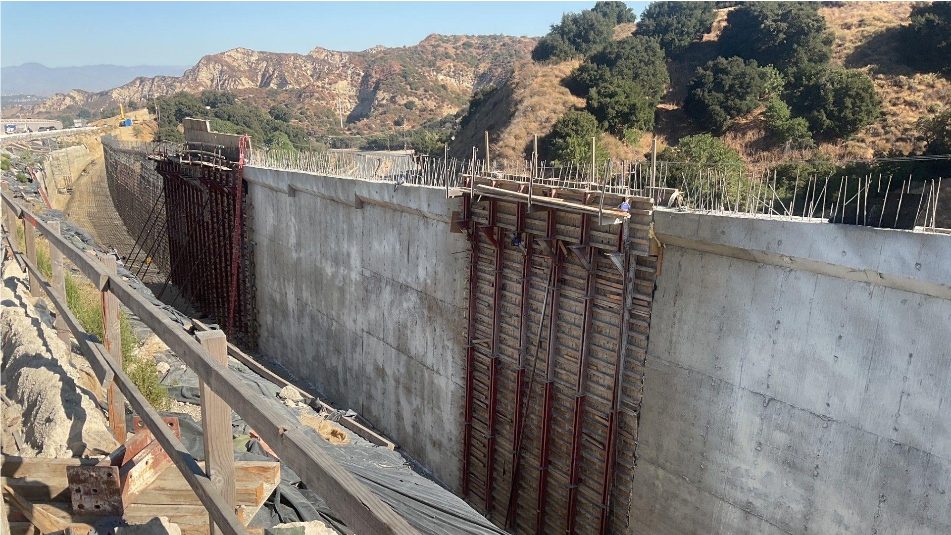
Retaining Wall between northbound Weldon Cyn Rd Bridge and Calgrove Bl off-ramp, September 2024
