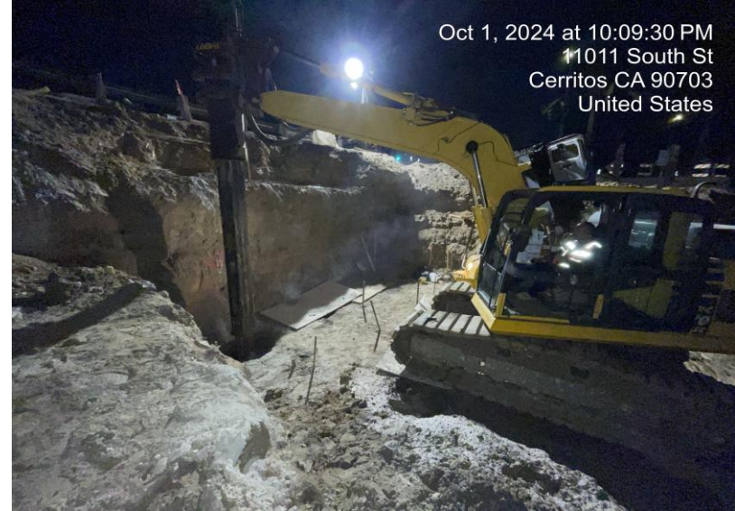
Drilling for pile installation for new retaining wall at South St SB off-ramp
