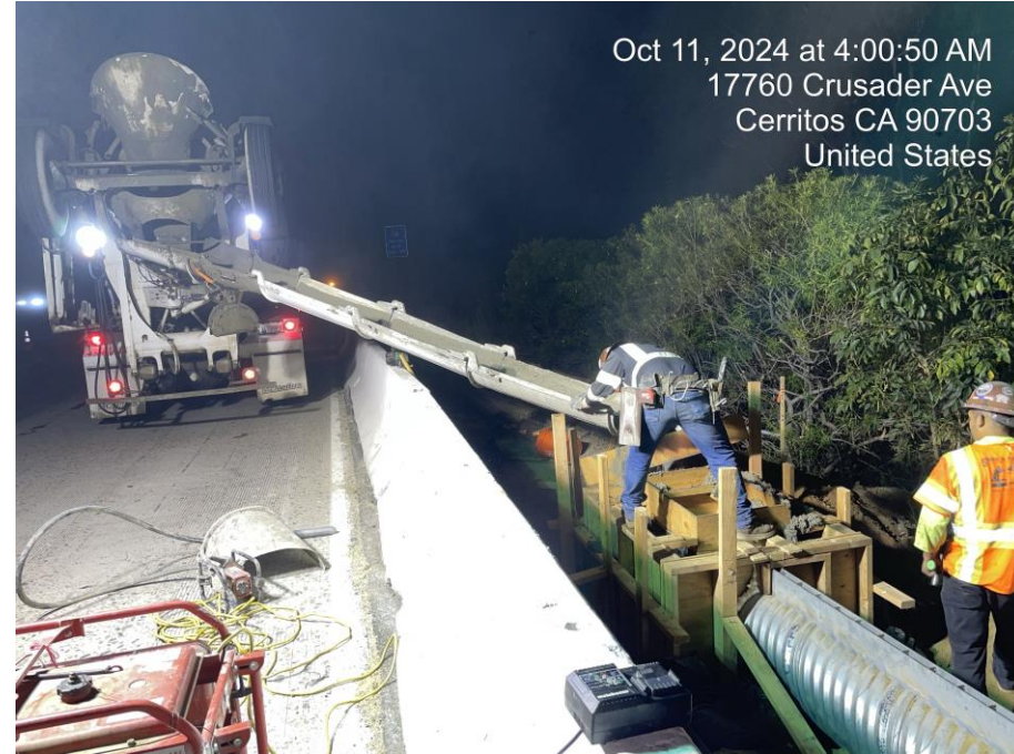
Concrete pour of inlet of new drainage system at South St SB off-ramp
