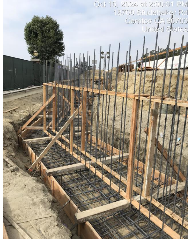
Rebar installation and forming of retaining wall at South St SB off-ramp
