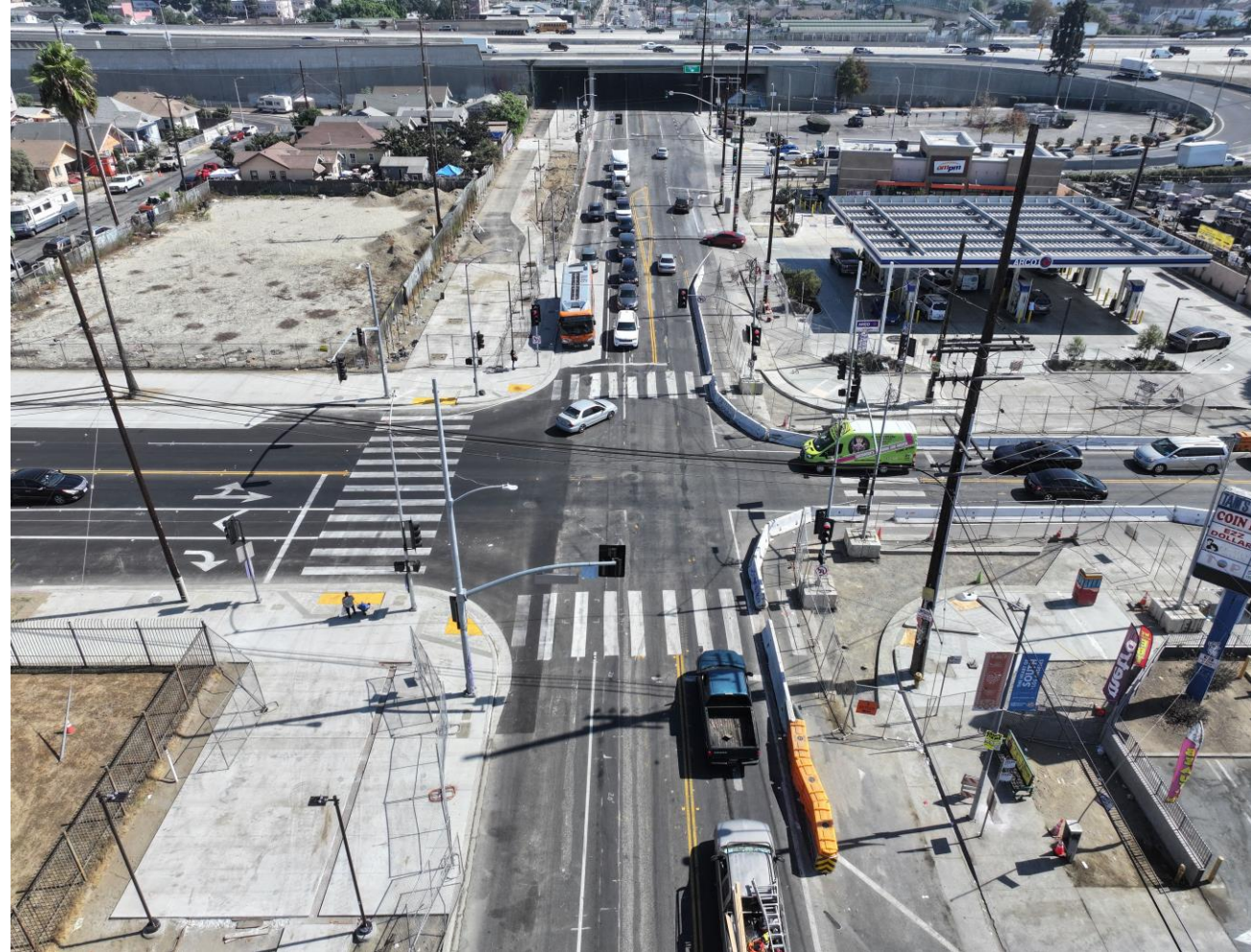
Reconstruction of the ADA Ramps on the south side of the Slauson/Figueroa Intersection
