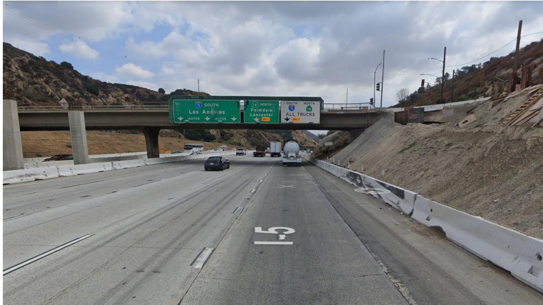
Existing sign structures on the Weldon Canyon Rd Bridge that will be replaced
