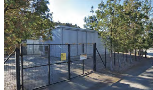
Traction Power Substation
