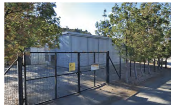
Traction Power Substation
