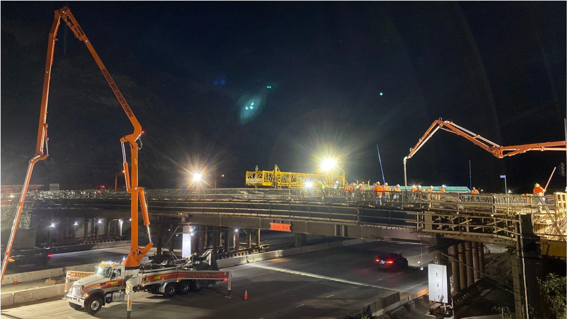
Concrete placement for the new deck on Weldon Canyon Rd bridge in May 2023
