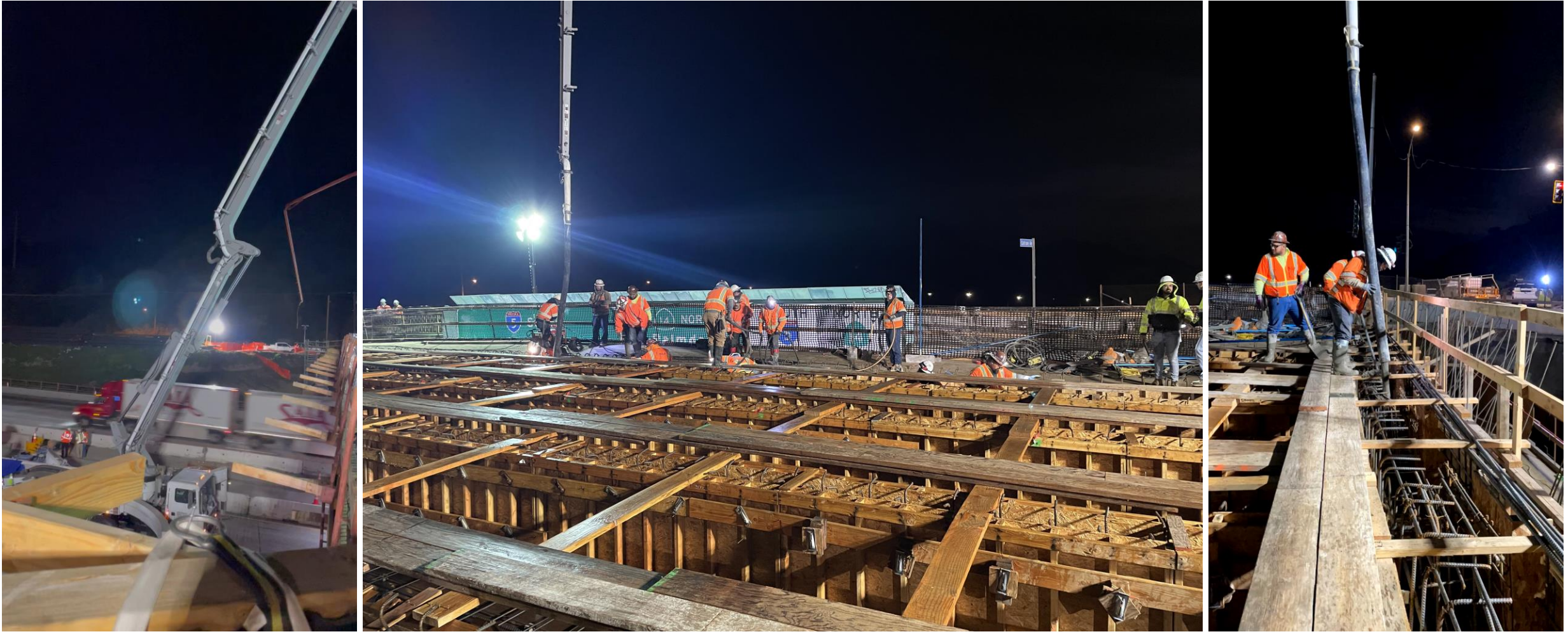
Concrete placement for the new Weldon Canyon Rd bridge in March 2023, with the use of lane closures on I-5
