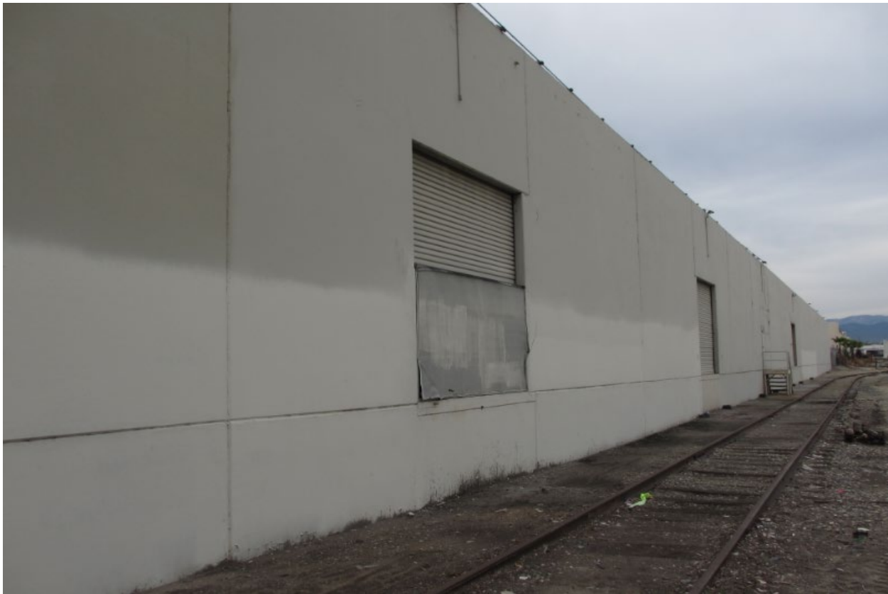
Figure 3.4.6. Goodyear Tire and Rubber Company Warehouse Constructed 1952 and Existing Rail Alignment Facing Washington Boulevard (2353 Garfield Avenue) (View east)
