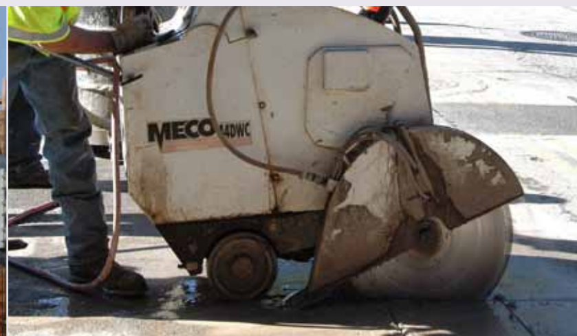
This crew cuts through the concrete of Ohio Av to pinpoint the location of underground electrical lines. The water on the street cools the saw and is vacuumed up later.
