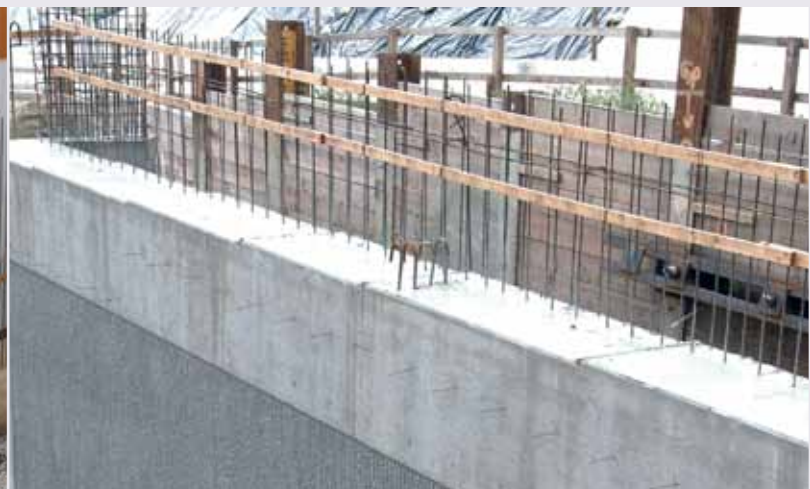
The newly poured west abutment of Sunset Bl Bridge. The area behind the wood supports will be backfilled with soil.
