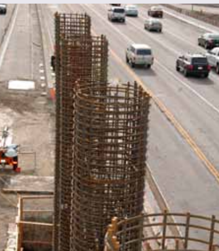
These round "cages," when surrounded in concrete, will become the center columns supporting Sunset Bl Bridge.
