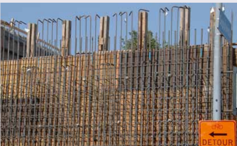
Looking south on Sepulveda Bl, this photograph captures the rebar that will become the extended support of the widened Montana Av bridge.
