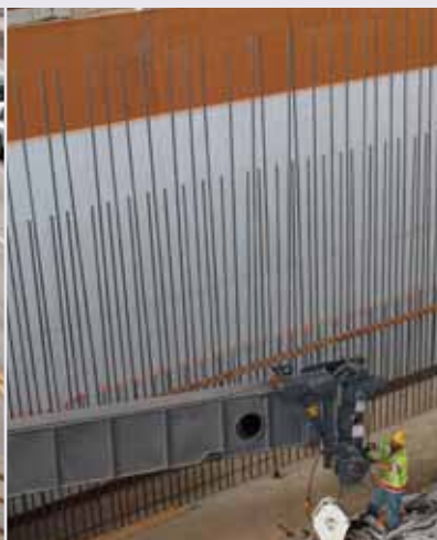
Workers install rebar to form the east abutment of Sunset Bl Bridge. A line of yellow impalement caps, seen behind the crane arm, protects workers.
